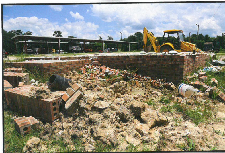
Old maintenance facility in Lake City before cleanup for recreational park development
